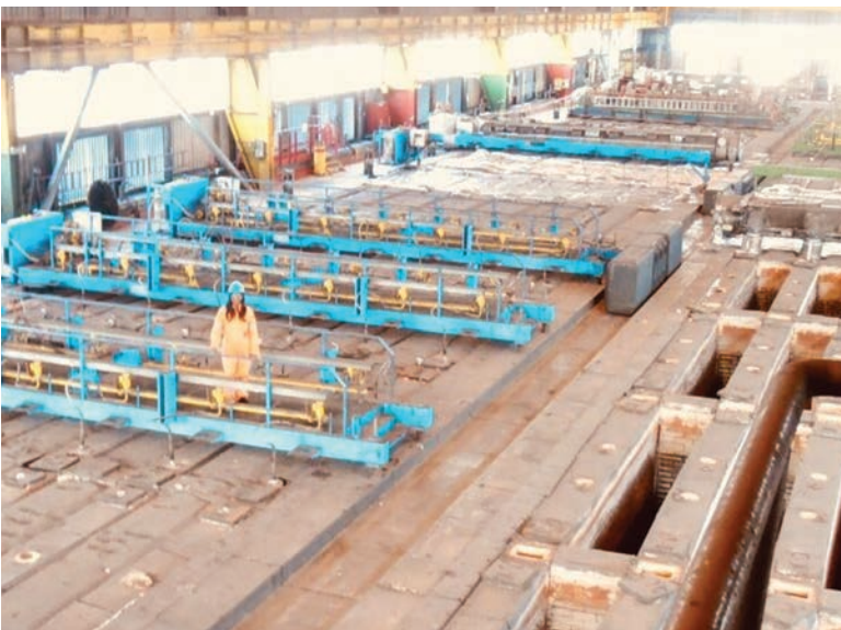
FIGURE 1 Anode baking furnace at Aluchemie.
